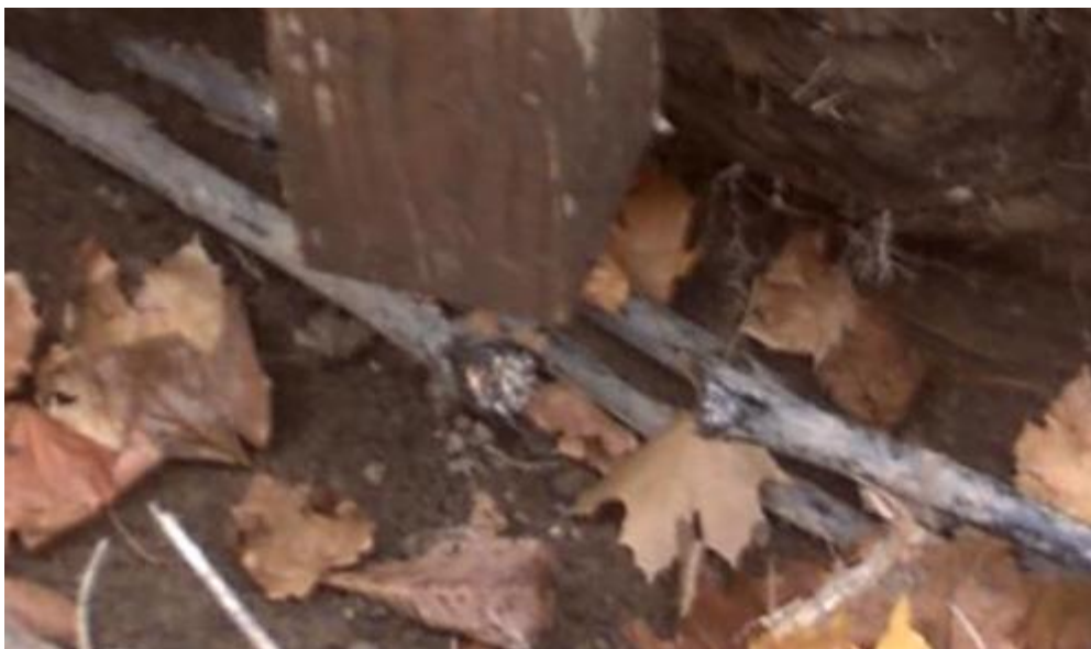
Photo 4 (close up of breach)
